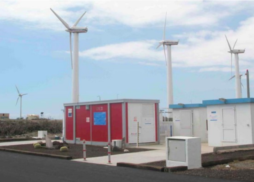
Wind generation plant with power set up to produce hydrogen on site as backup storage system
