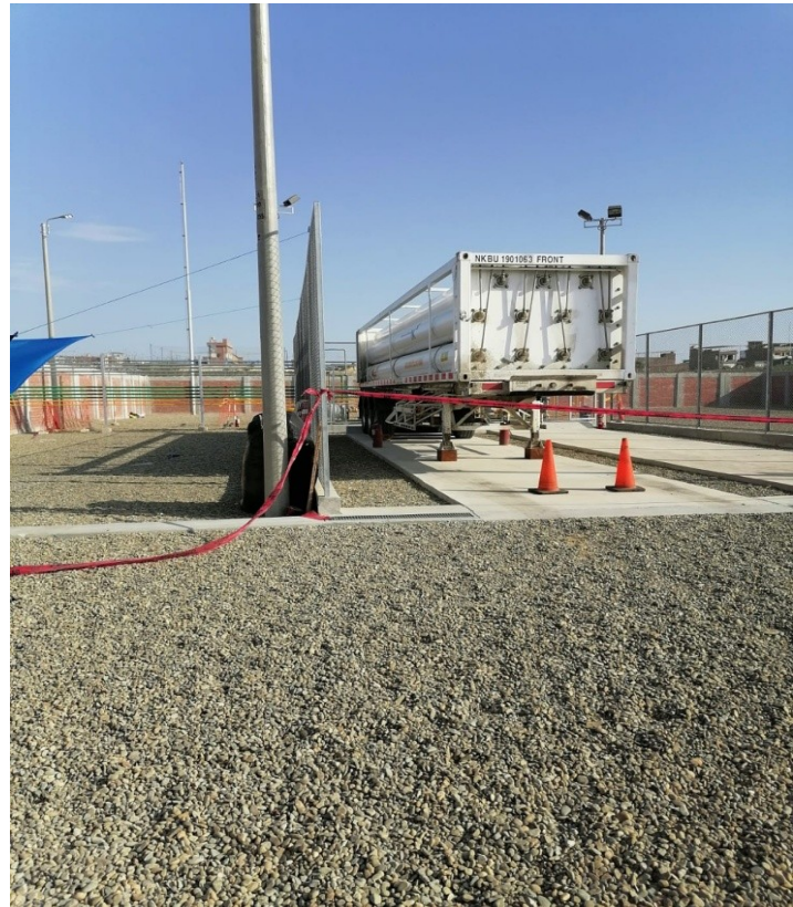
LPG power supply plant with atmospheric lightning rod protection
